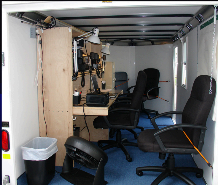
Mobile Communications Trailer
