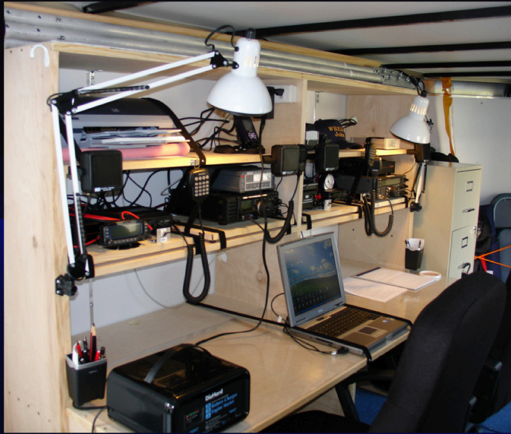
Mobile Communications Trailer
